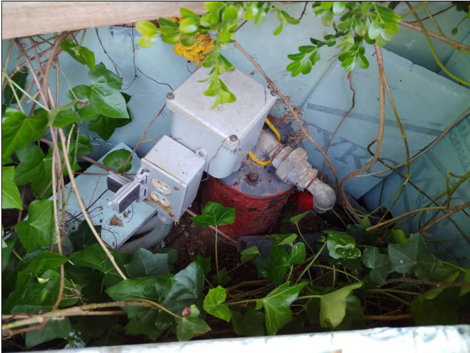
Photo C3: Looking down and east at the stick-up and well head configuration for Well 64284 (Observation Well)
